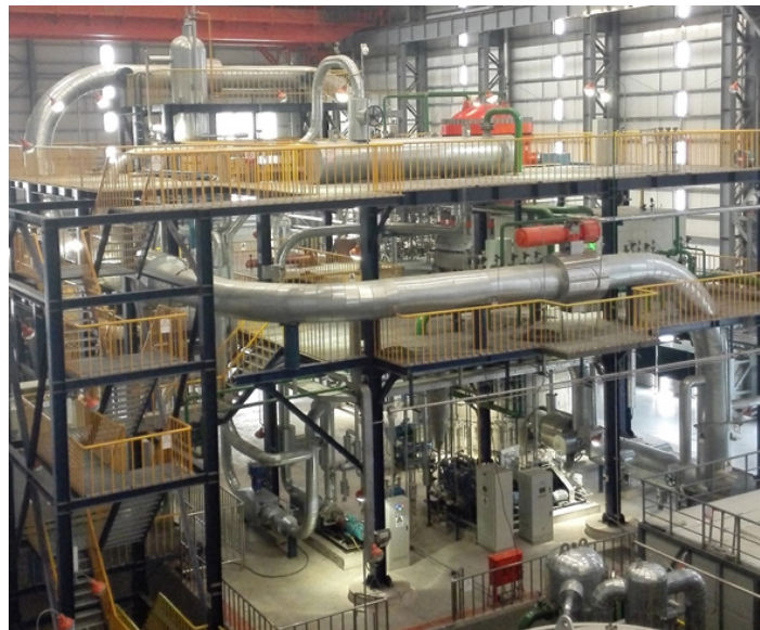
Figure 3.53: Engineering test facility of main helium circulator (ETF-HC) at INET's HTR-PM Laboratory
